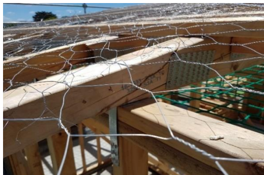
Broken trusses not allowed to be fixed by anyone but Truss Company
